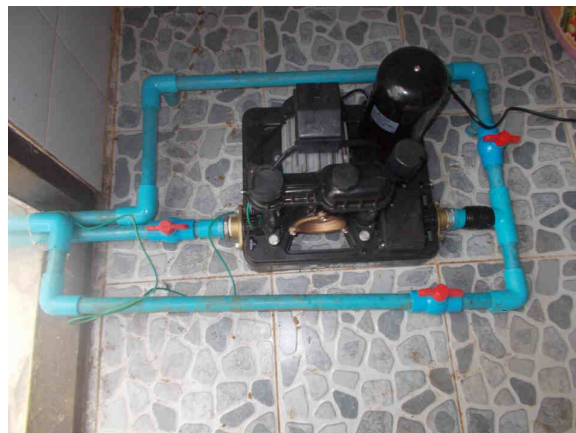
The new water pump
