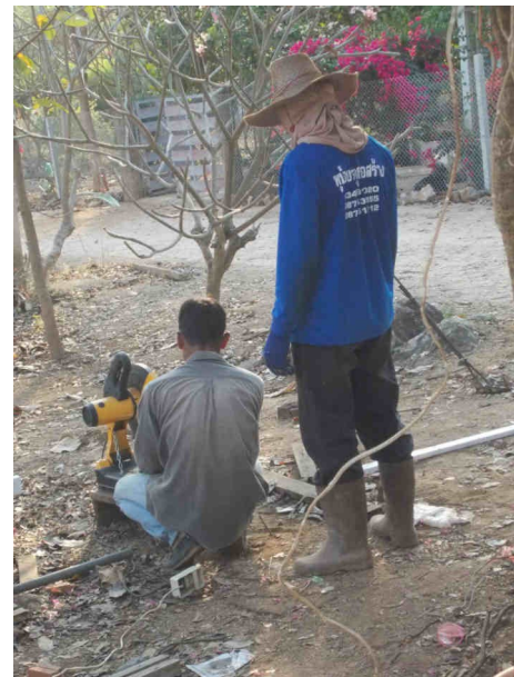
Khun Ekgarat (left) und Khun O cut steel girders for the roof.
